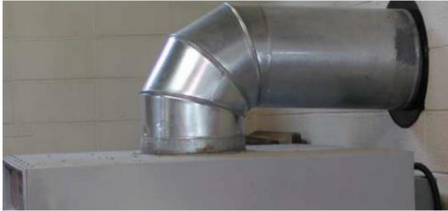
Figure – Ducting from Top of Cabinet
